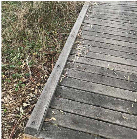
Image 11: Kickrail used on all boardwalks for wheelchair safety
