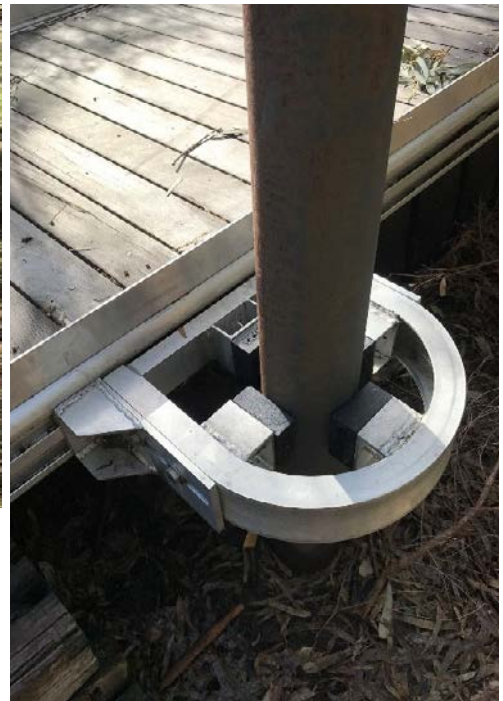
Image 15: Pontoon style boardwalk anchoring pile
